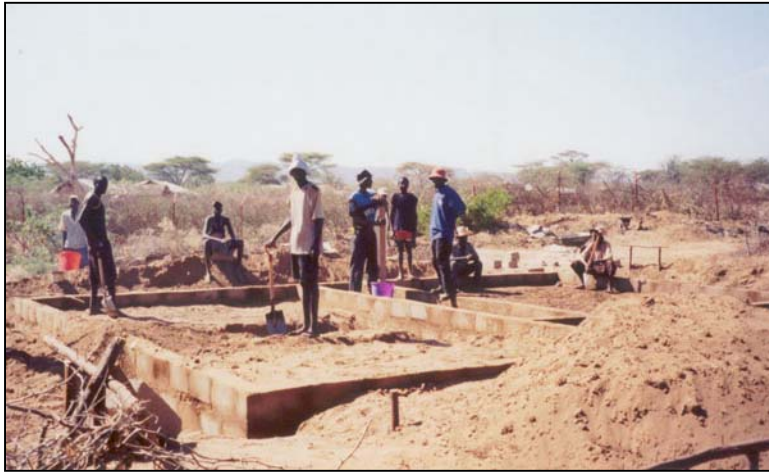
Refugee workers hired to help in the construction of a building in the camp
